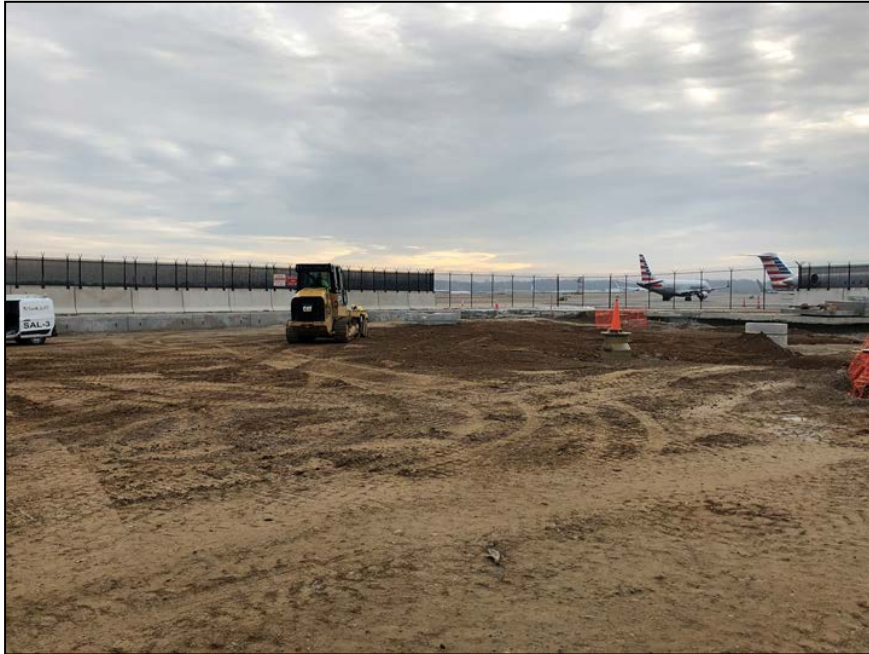
North/South Trench Drain
