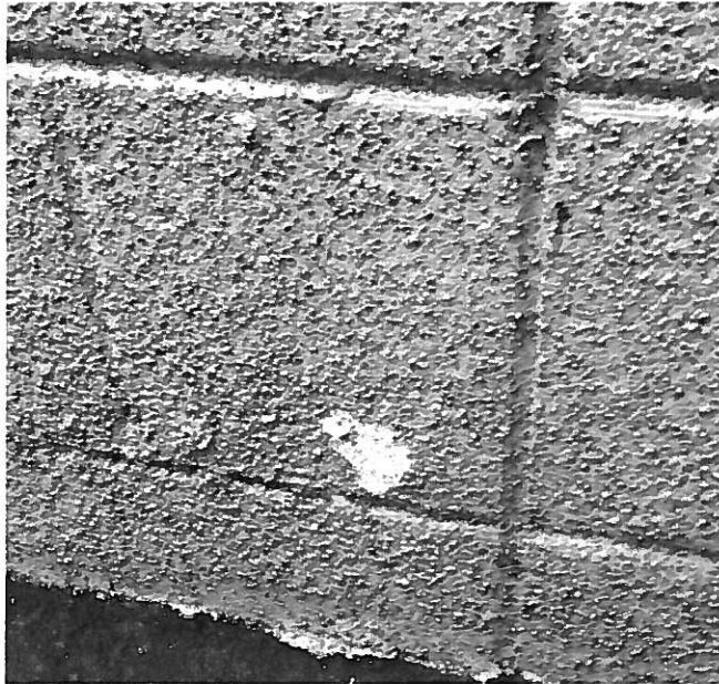
37. Non-ACM exterior textured surfacing wall coating (TW1-Samples 132, 133, 134, 135, 136, 137, 138) on the exterior wall of the building.
