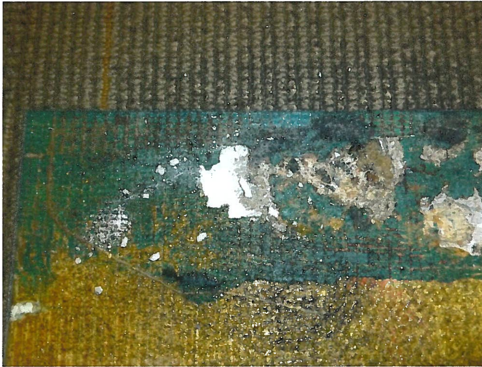
11. Non-ACM gray leveling compound beneath 2' x 2' carpet squares (LV1-Samples 25, 26) in hall outside Office 180.18.
