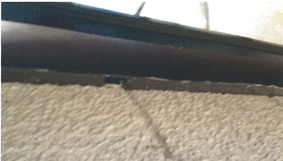
34. Non-ACM brown exterior window caulking (CK4-Samples 126, 127) on the exterior windows of the building.
