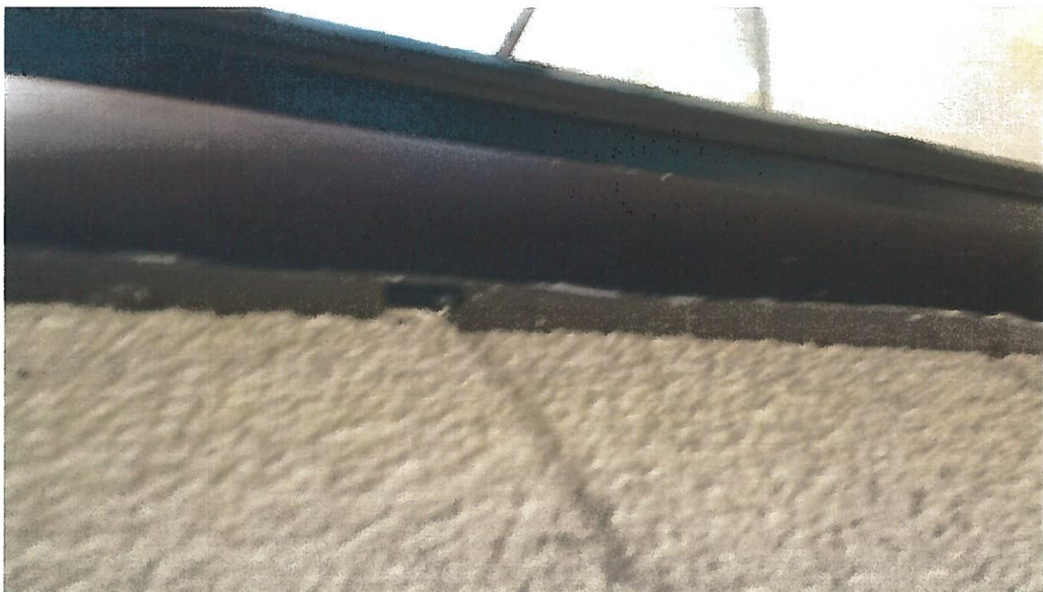
34. Non-ACM brown exterior window caulking (CK4-Samples 126, 127) on the exterior windows of the building.
