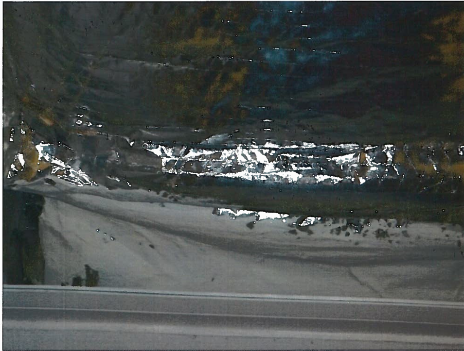
41. Non-ACM white seam mastic on foil fiberglass duct insulation (SM7-Samples 147, 148) in 225.00 Bridge to hangar.
