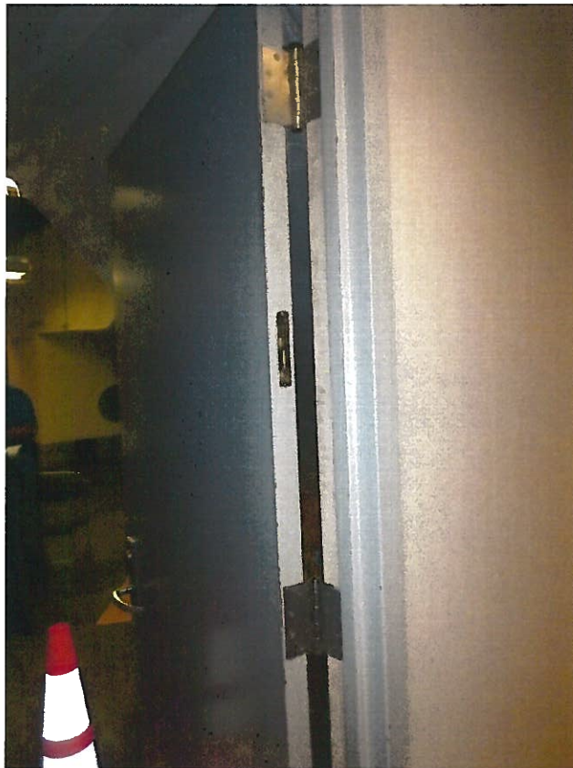
52. Assumed ACM fire door (no samples collected) at Mechanical Room 263.01.
