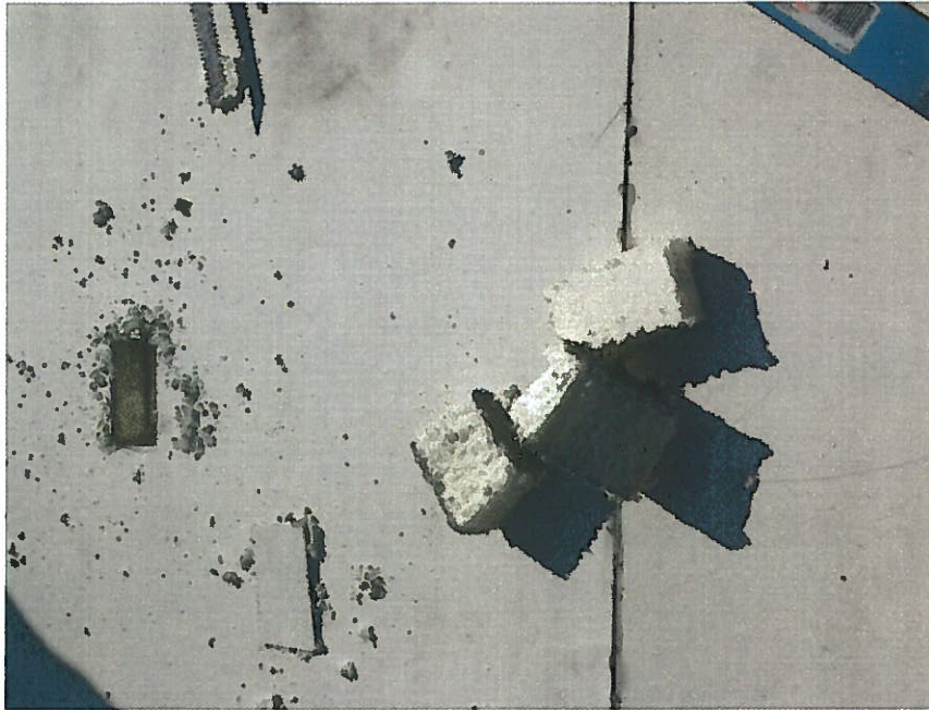
51. Non-ACM felt paper between foam roofing layers (RFL2-Samples 167, 168) on the exterior roof of building – addition portion.
