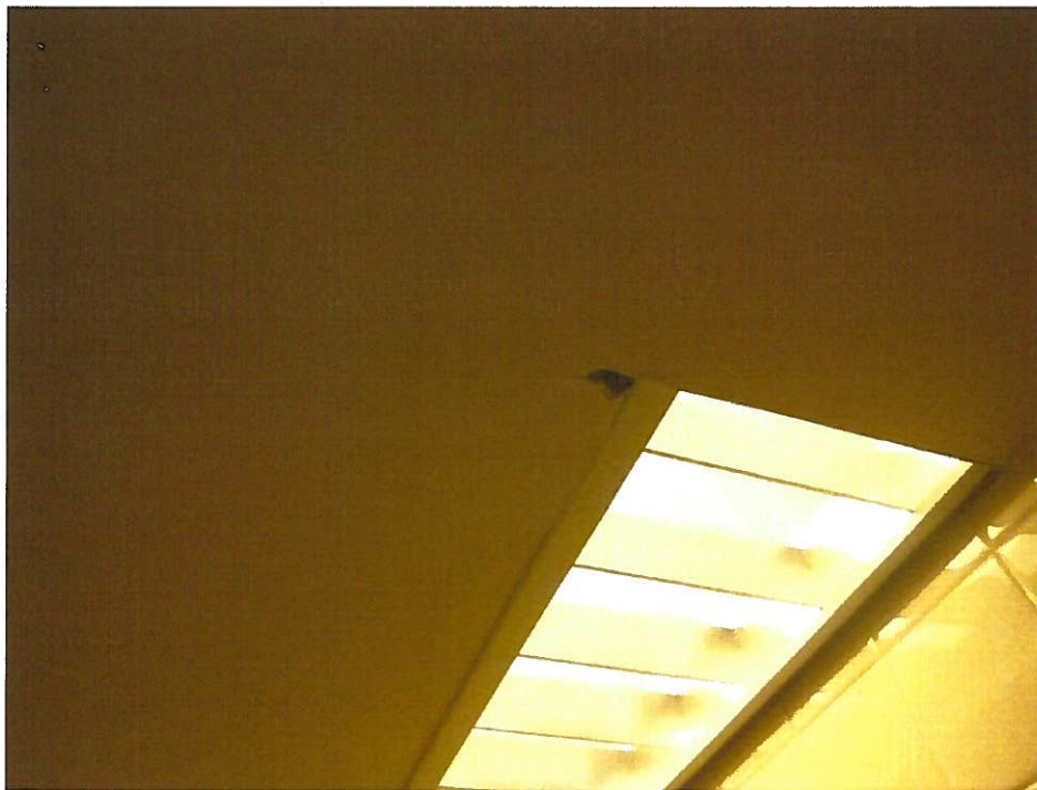
24. Non-ACM gypsum ceiling board with joint compound (DJ4-Samples 74, 75) in Men's Restroom next to 102.
