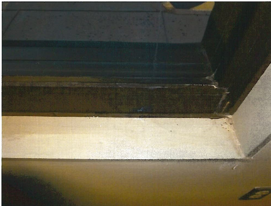
12. Non-ACM beige interior window frame caulking (CK1-Samples 27, 28) and brown interior window caulking (CK2-Samples 29, 30) in Office 188.20.
