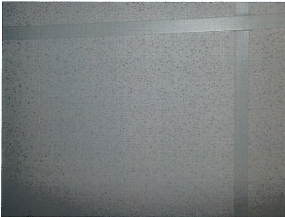
28. Non-ACM 2' x 2' pinhole and small gouge ceiling tile (CT3-Samples 94, 95) in Reception 138.09.
