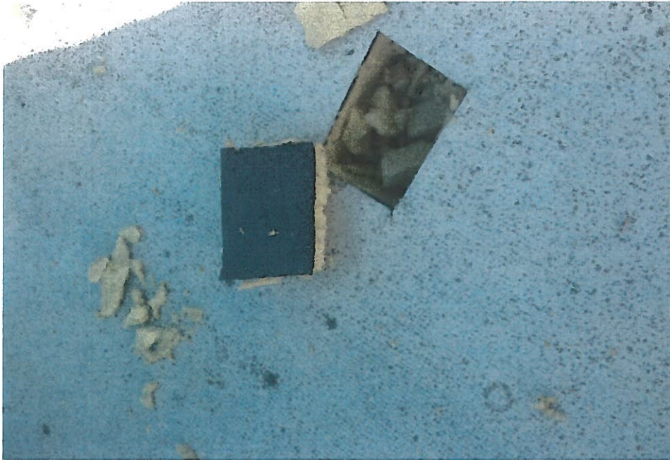
47. Non-ACM felt paper between foam roofing layers (RFL1-Samples 159, 160) on the southwest roof of the building.
