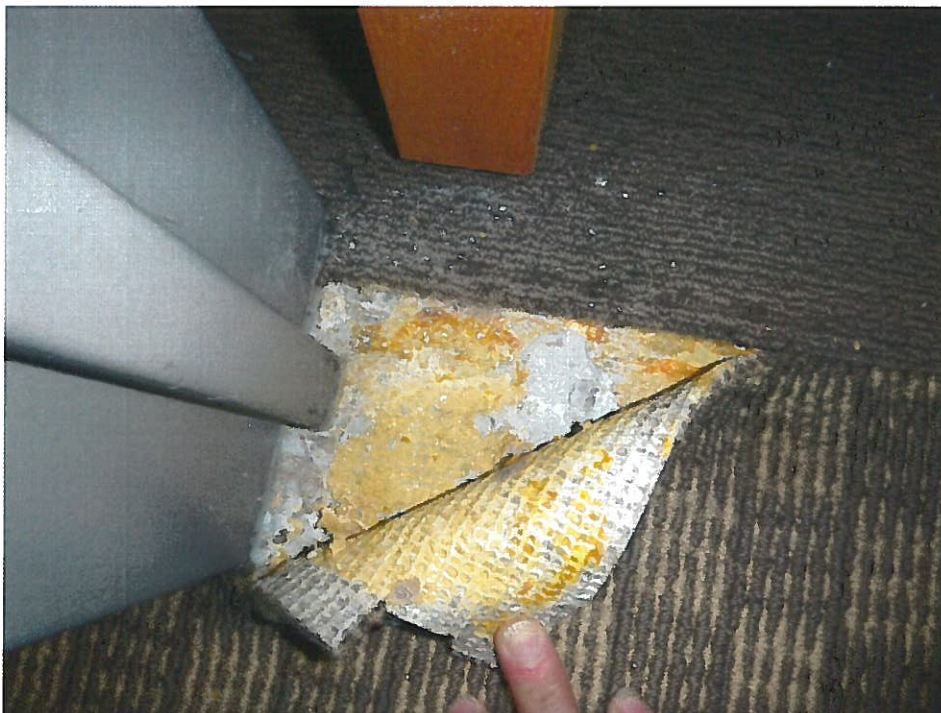
46. Non-ACM gray leveling compound (LV2-Samples 157, 158) beneath carpeting and carpet mastic throughout the third floor.
