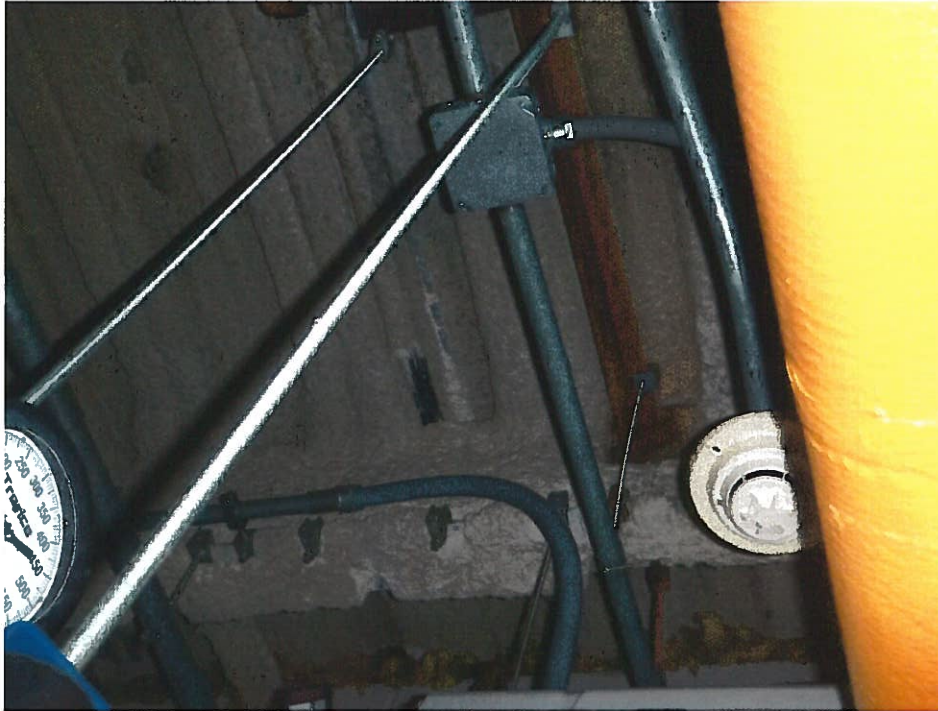
13. Non-ACM spray-on fireproofing on metal rolled ceiling deck and columns (2 layers – FP1-Samples 31, 32, 33, 56, 57 and FP2-Samples 38, 39, 40, 41, 42, 114, 115) throughout the building.
