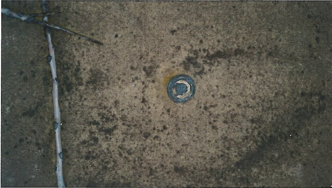
Photograph of 2" suspect fill port located within Open Area 104 of the Corporate Office Building. Use of the fill port is unknown; may be associated with former or abandoned oil filled equipment.
