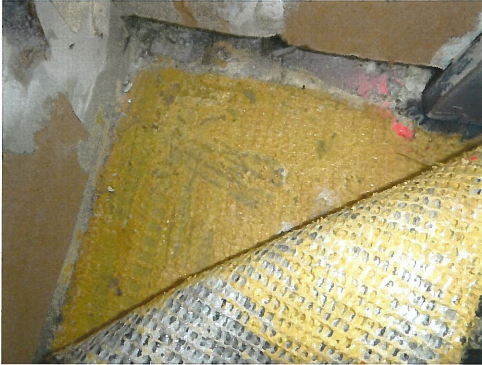
43. Non-ACM yellow mastic beneath rolled carpeting (CM3-Samples 151, 152) in Office 310.
