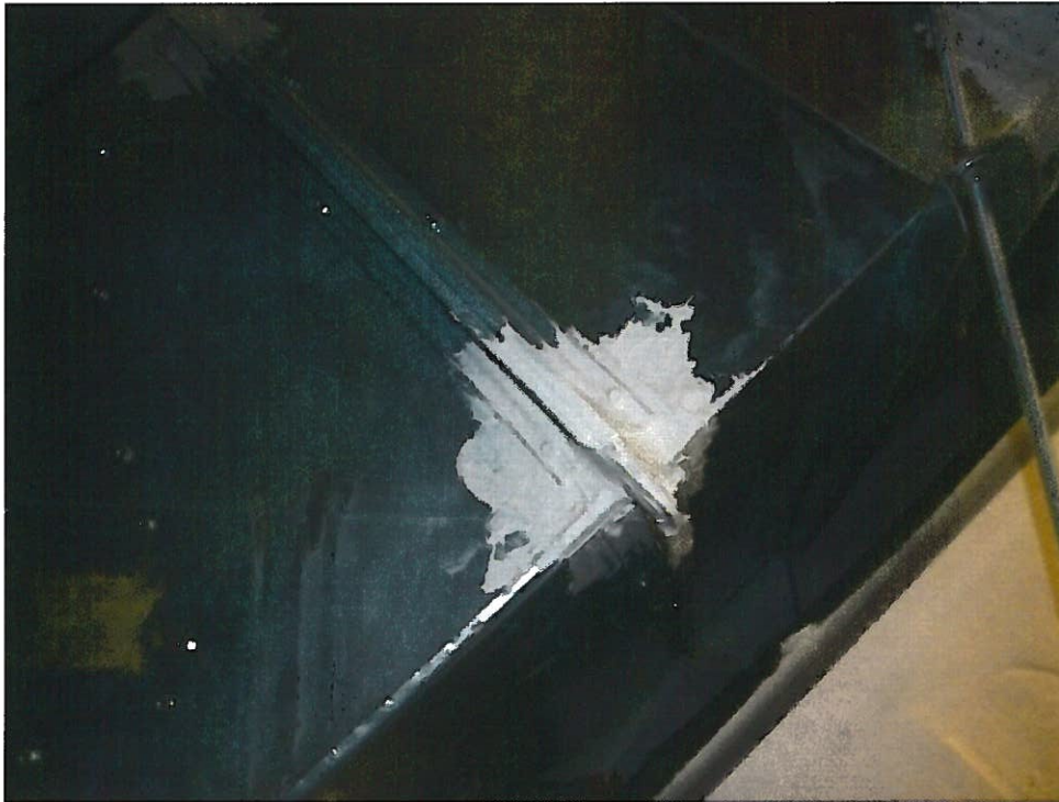
5. Non-ACM white seam mastic on metal ducting (SM5-Samples 11, 12) in Mechanical Room 263.01.
