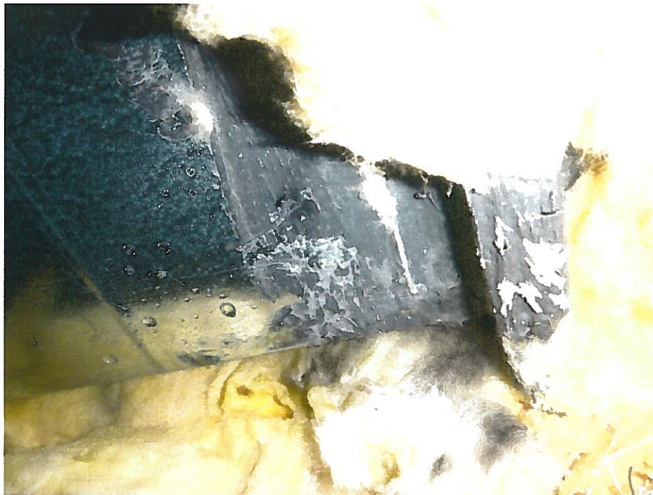
2. Non-ACM gray seam mastic on metal ducting (SM3–Samples 05, 06) above drop ceiling in the hallway outside Office 180.18.
