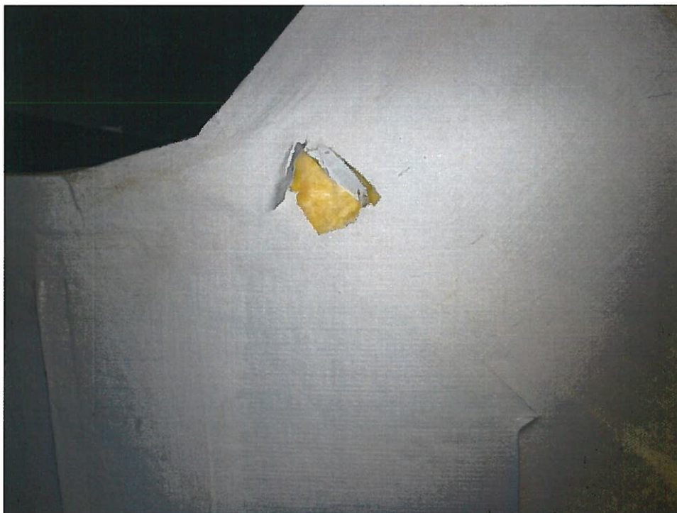
4. Non-ACM white mastic on white fiberglass duct insulation (SM4-Samples 09, 10) in Mechanical Room 263.01.
