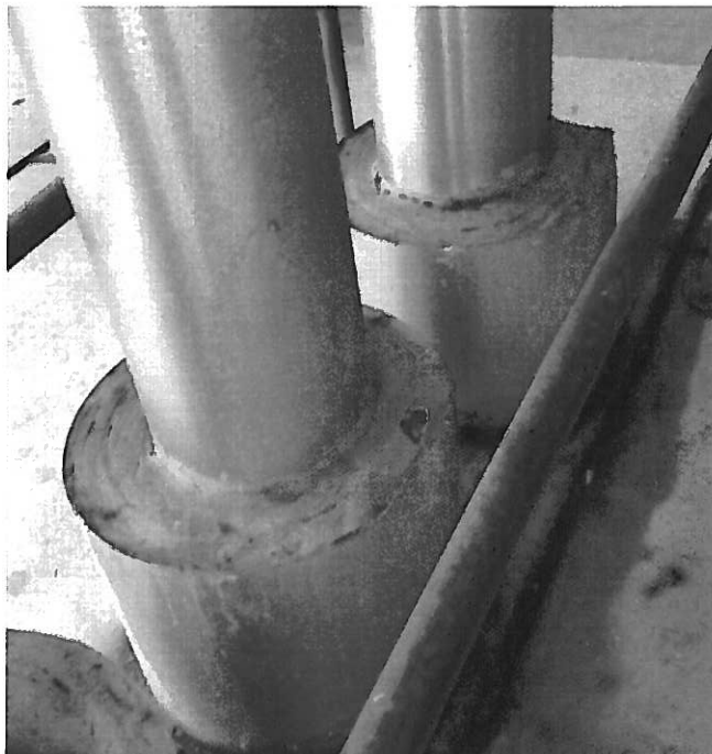
38. Non-ACM end cap mastic on exterior piping (ECM3-Samples 139, 140) on the exterior north side of the building.
